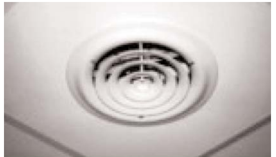
▲ Typical outlet grill
