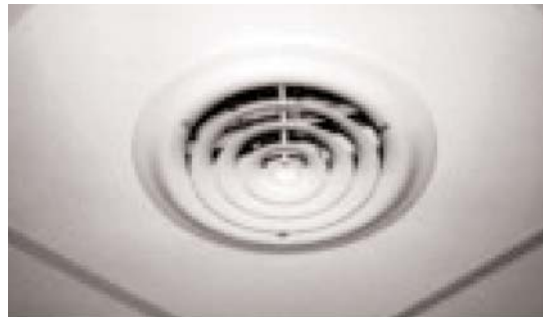
▲ Typical outlet grill
